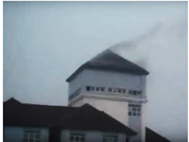
Figure 16 Screen grab of the smoldering roof of one of the building's two water tank towers soon after the lightning strike in April 2010
