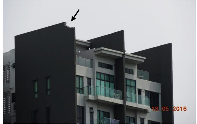
Fig. 2.5. A much larger bypass on top of a firewall. The same bypass shown in fig. 2.4 had been repaired earlier.
