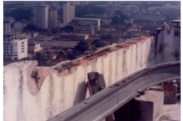
Fig. 2.6. A very large bypass on the parapet wall, photographed in 1991. The building had just been installed with a CVM air terminal.
