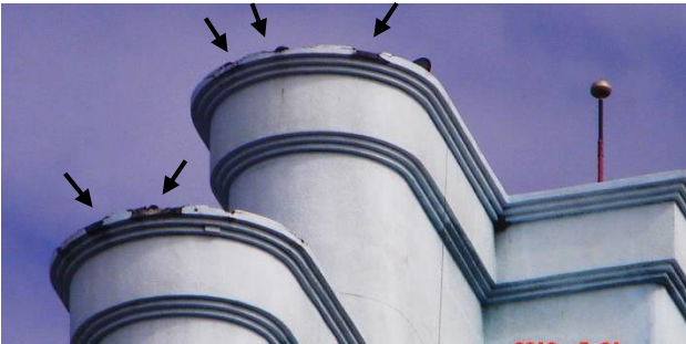
Fig. 4.3. Multiple bypasses were observed on the lower level parapet walls located near the CVM air terminal.
