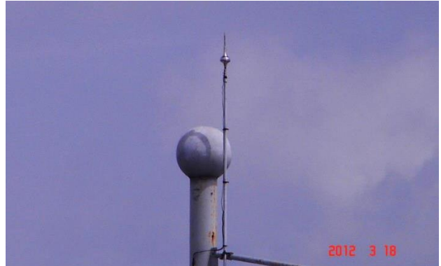
Fig. 5.5. The ESE air terminal mounted on one of the grandstand's metallic pillars.
