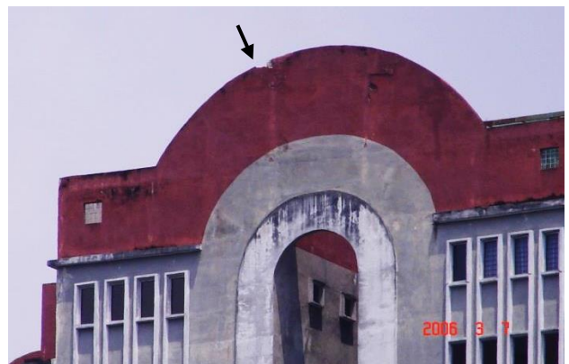
Fig. 2.8. A bypass on top of a curved facade.
