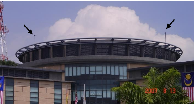
Fig. 4.4. Two second generation CVM air terminals (arrowed) installed on a low-rise public building.
