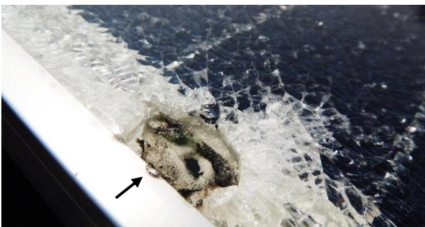
Fig. 5.3. One of the bypasses located at the edge of the solar panel. The blob of melted metal (arrowed) on the aluminum frame suggests that it was caused by a very high temperature event, such as a lightning stroke.
