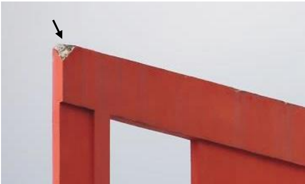
Fig. 2.2. A small bypass on top of a facade with the lightning impact point at the wall end.
