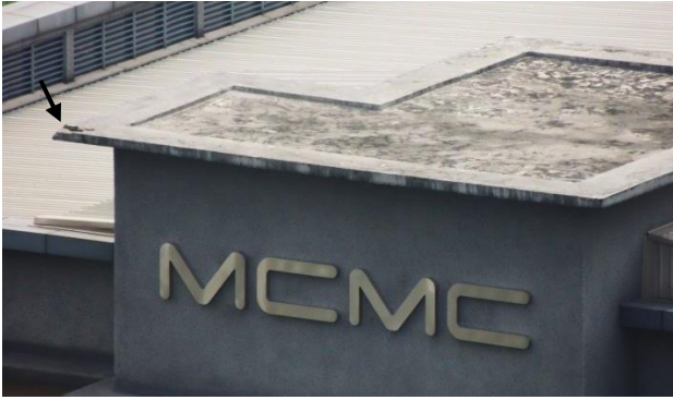
Fig. 2.1. A small bypass located at the corner of the roof of a public building. This is the most common shape of bypasses seen in Malaysia.
