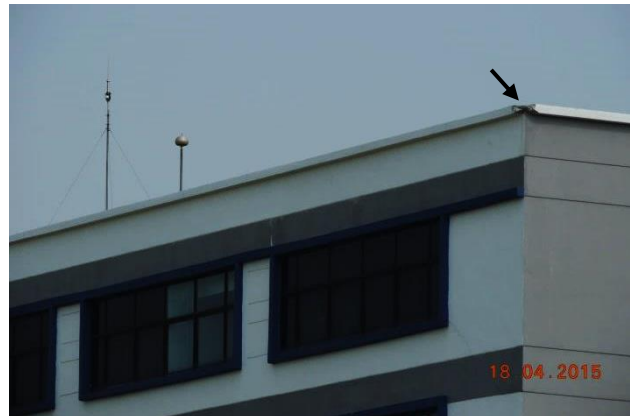
Fig. 4.8. The same building observed with a bypass (arrowed) in 2015.
