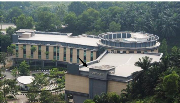
Fig. 4.5. A bypass was observed on the corner of the roof (arrowed). See fig. 2.1 for a close-up picture of the bypass.
