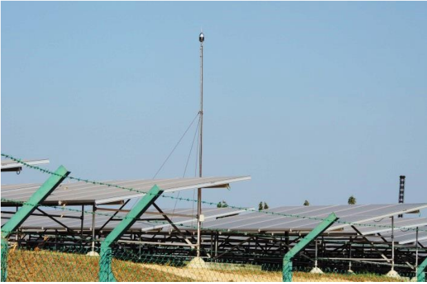
Fig. 5.1. One of several mast-mounted ESE air terminals installed at a photo-voltaic farm where a bypass had occurred.
