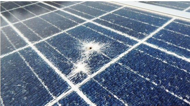
Fig. 5.2. Two of the bypasses on the center portion of a solar panel that was struck by lightning.
