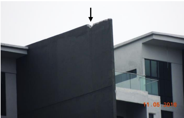
Fig. 2.3. A small bypass on top of a firewall with the lightning impact point located away from the wall end.
