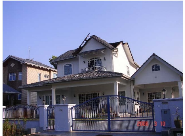
Fig. 1: The damaged roof of a house that was struck by lightning.
