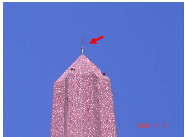
Fig. 6: An ESE air terminal on the apex of the minaret (arrowed).
