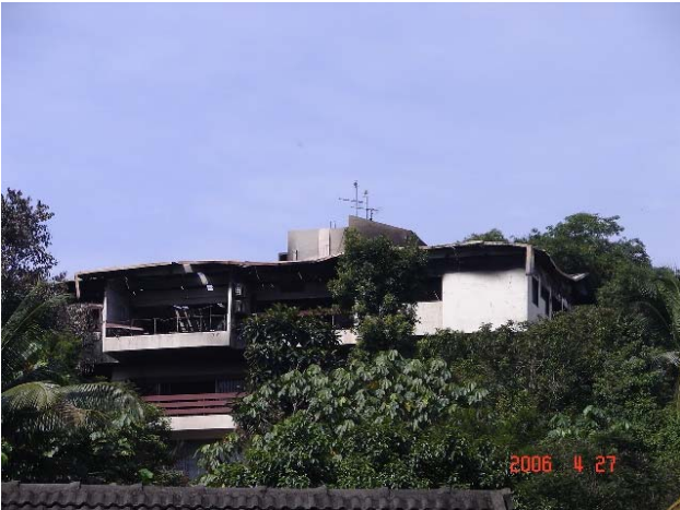
Fig. 3: The fire damaged top floor of a house that was struck by lightning.
