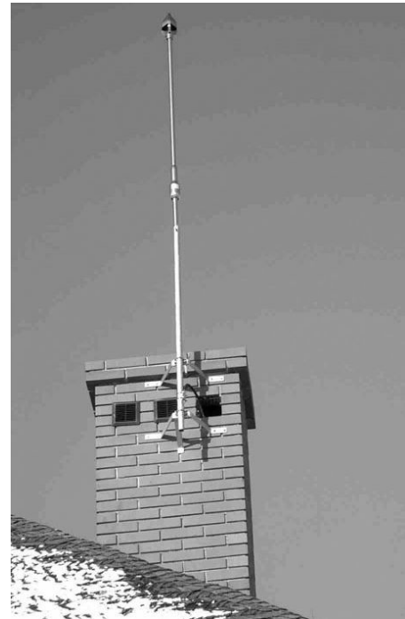
Fig. 8. Stupid advertisement (www.megatech.com.pl): a down conductor coming into a “protected” house
